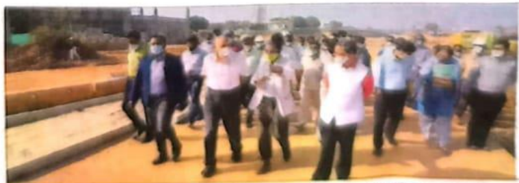
Chief Secretary P Ravikumar inspects the ongoing works at the permanent campus of IIT-Dharwad during his visit to Dharwad recently. IIT-Dh director P Sheshu, Deputy Commissioner Nitesh Patil and others are seen. DH PHOTO
